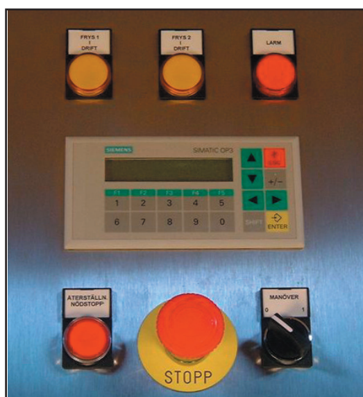
Example of a control unit
